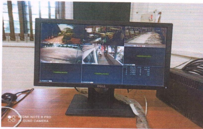
CCTV Monitoring Screen
